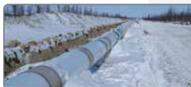
Completed Skin Trace system prior to burying
